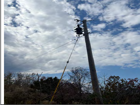
Overhead transformer. No leaks or stains noted.
